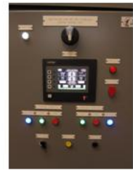
4: Local control unit
